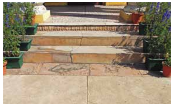
Pic 14: Damaged steps of western portico
