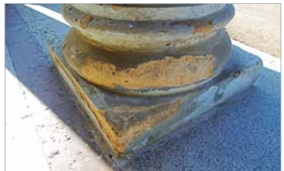
Pic 21: Flaked plaster on columns
