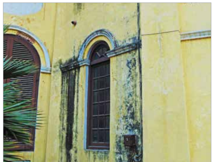
Pic 24: Black spotting and flaking on mouldings
