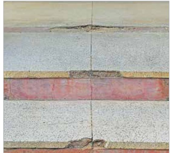
Pic 25: Damaged entrance steps
