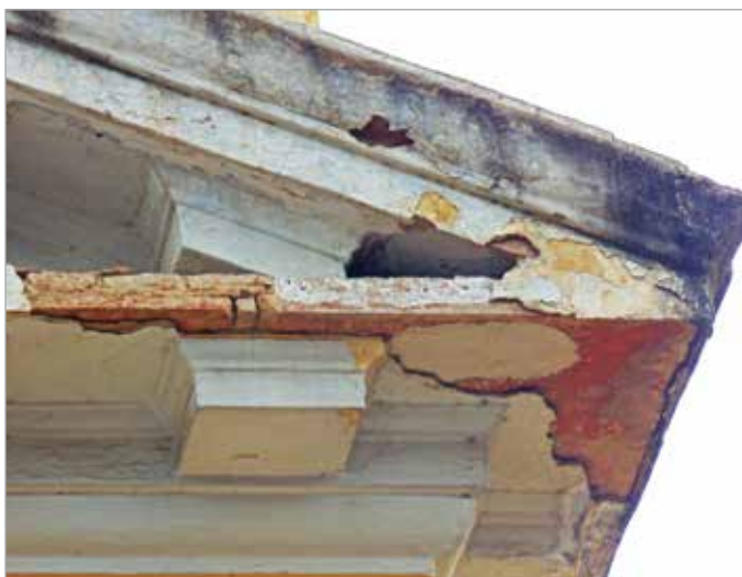
Pic 23: Damaged cornice mouldings
