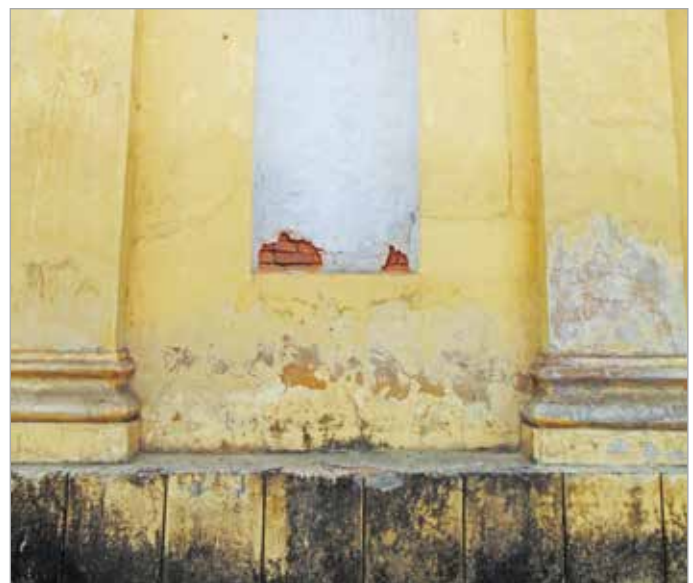
Pic 28: Black spotting and damaged plaster on pilasters and plinth surface
