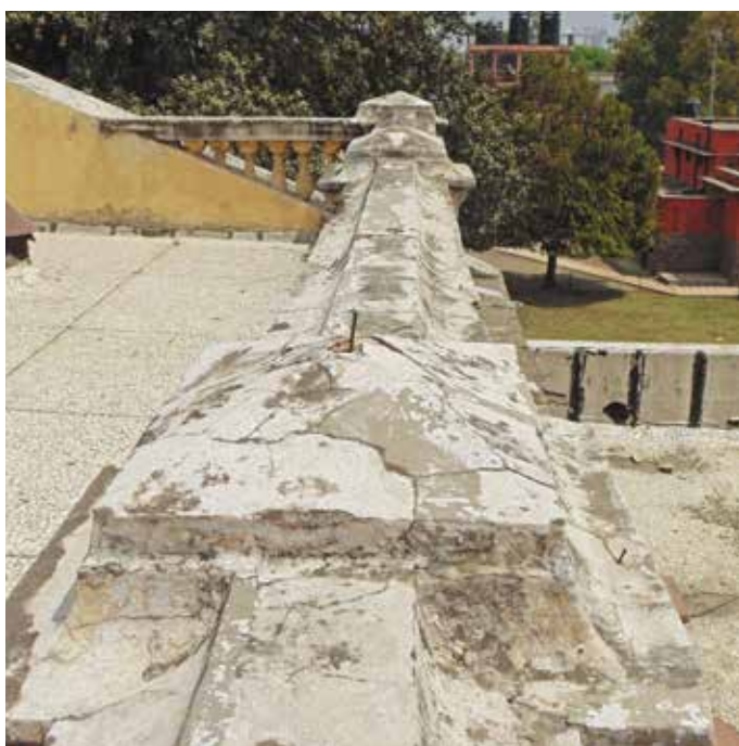
Pic 10: Damaged surface of parapet wall
