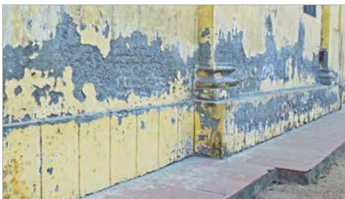
Pic 18: Damaged plaster and on walls
