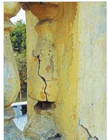
Pic 09: Damaged balusters
