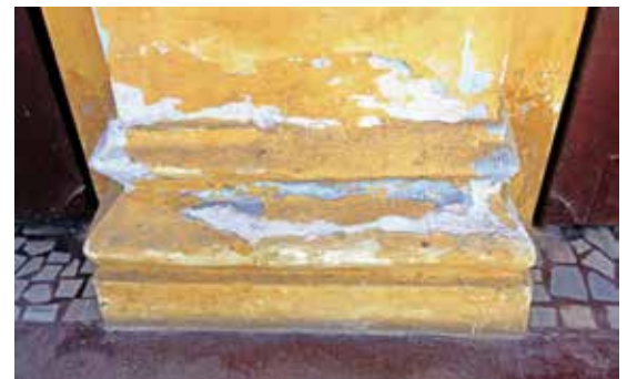
Pic 13: Damaged lime-wash on walls
