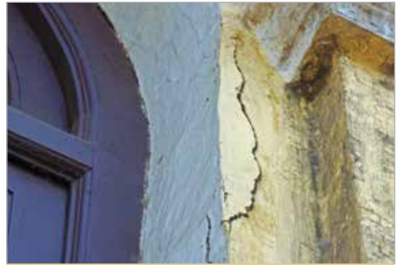
Pic 20: Cracked plaster of walls
