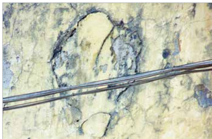
Pic 17: Bulging of plaster
