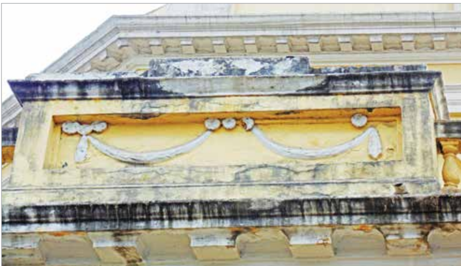
Pic 08: Black spotting on parapet and disfigured mouldings
