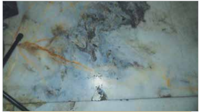
Pic 07: Staining of marble flooring near Lactern
