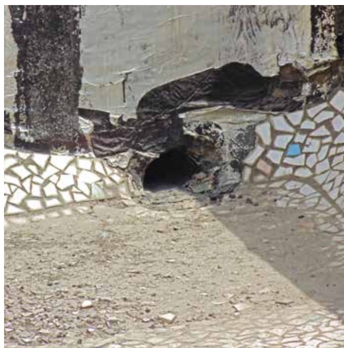
Pic 11: Blocked rain water pipes
