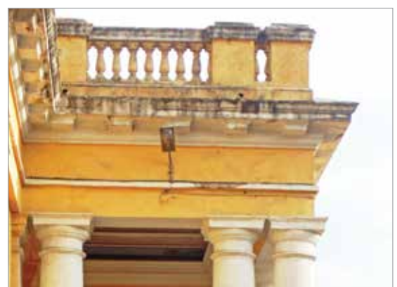
Pic 15: Black spotting and dampness on wall and moulding surface
