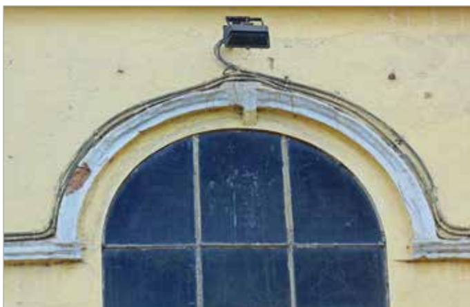
Pic 16: Damaged mouldings due to exposed electrical conduiting and fixtures
